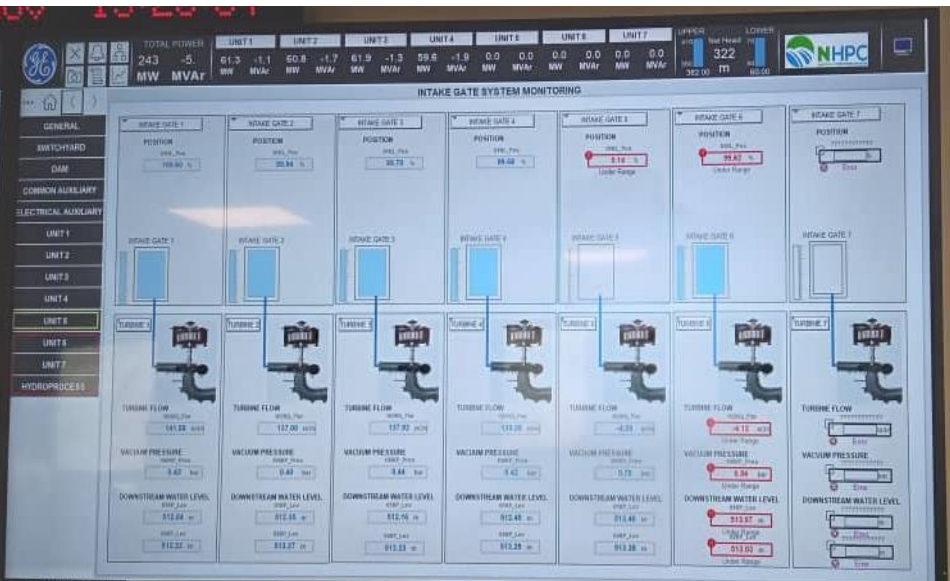
A picture of the Nachtigal hydroelectric facility's control screen
