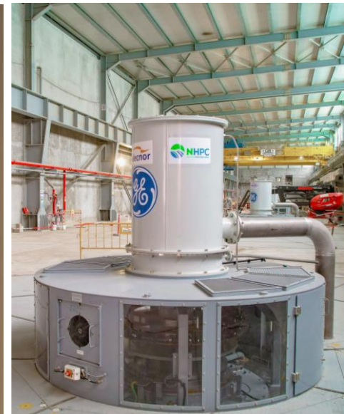
A picture of the Nachtigal hydroelectric facility's Unit No. 4
