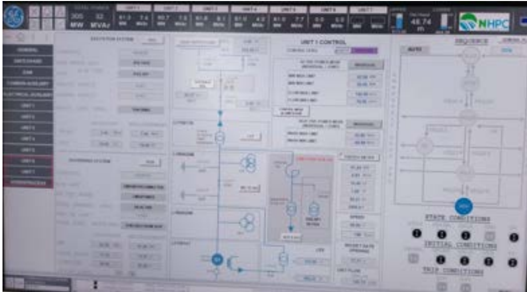
Photo of the Nachtigal hydroelectric facility' control screen
